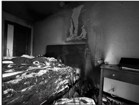
In a June fire near Suquamish, a closed door between this bedroom ...
